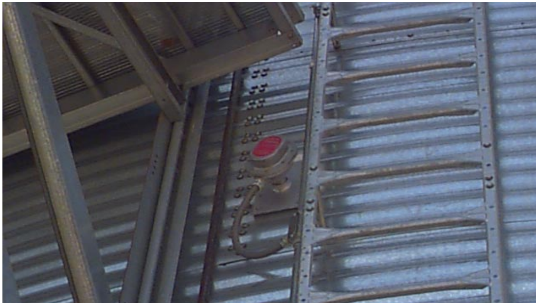
Storage chamber rotary switch.
